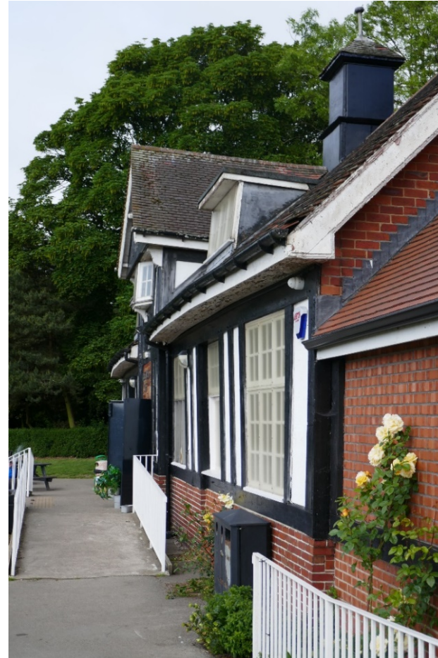
Photo looking west along the south facing front elevation showing the bowing out and leaning in the front wall and roof line to the front façade. Also note the dormers leaning back into the snagging roof line.
